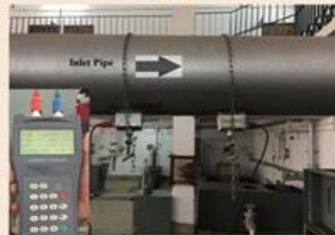
Discharge measurement using Ultrasonic flow meter
