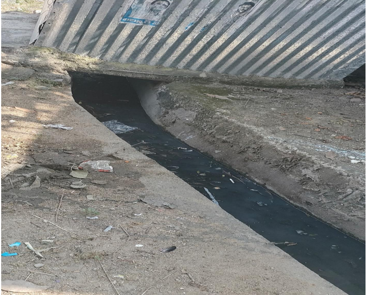
Picture 3: Stagnation of water due to blockage and poor design
