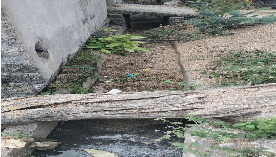
Picture 4- Blocakage of drain due to accumulation of silt and poor gradient design
